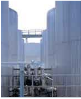
Storage tanks on the Belgian site
